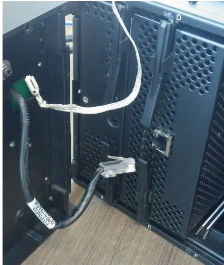
Figure 8-16: Disconnected ground cable and CPU connector
