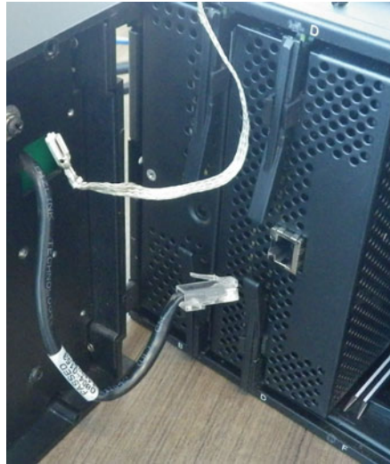
Figure 9-16: Disconnected ground cable and CPU connector
